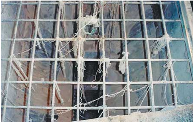
The grate size above this loading hopper should be reduced to prevent material from falling into the mixing area.
