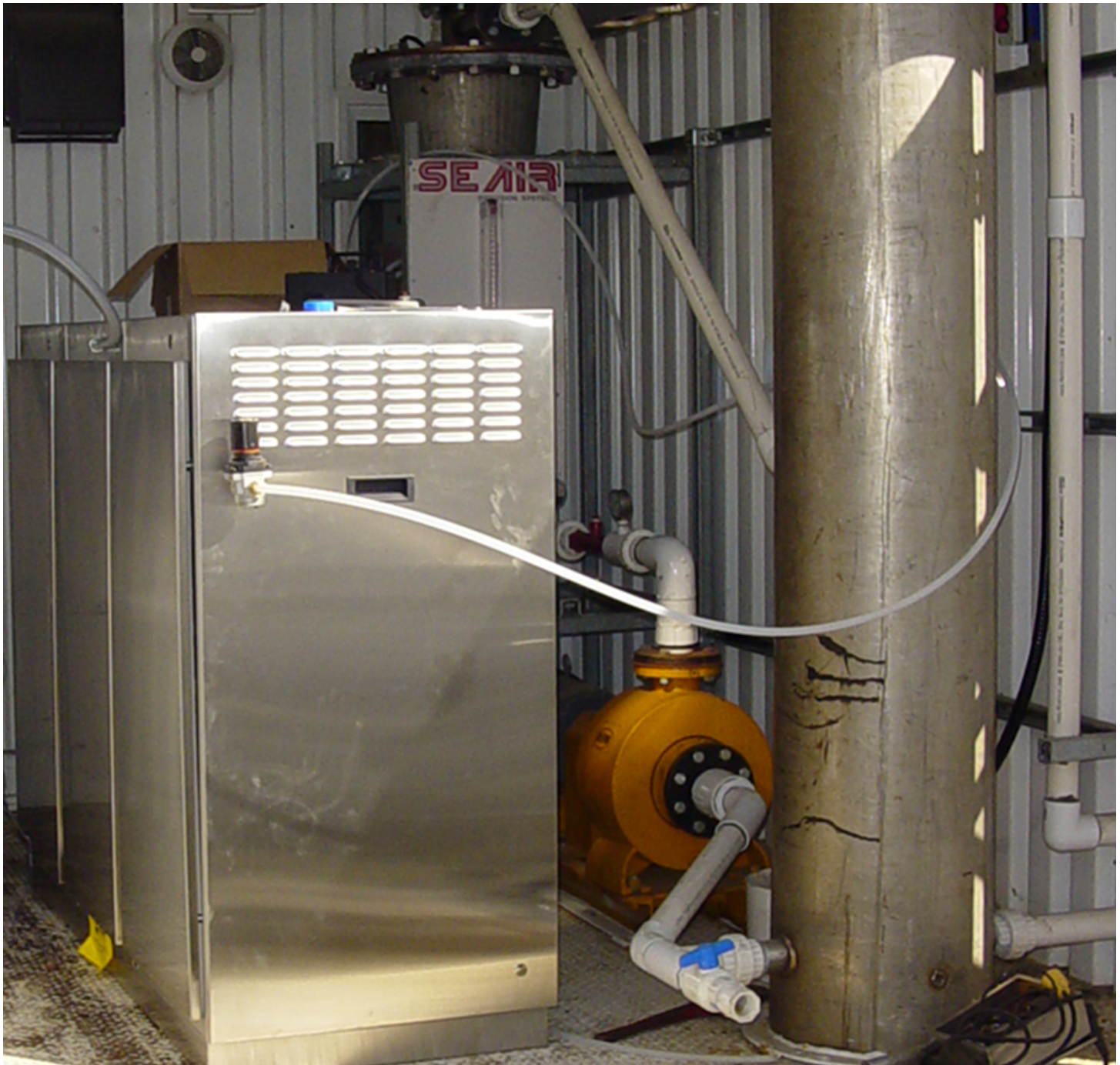
Ozone systems effectively treat wastewater from seafood processing plants. Photo courtesy of Pacific Ozone Technology.
